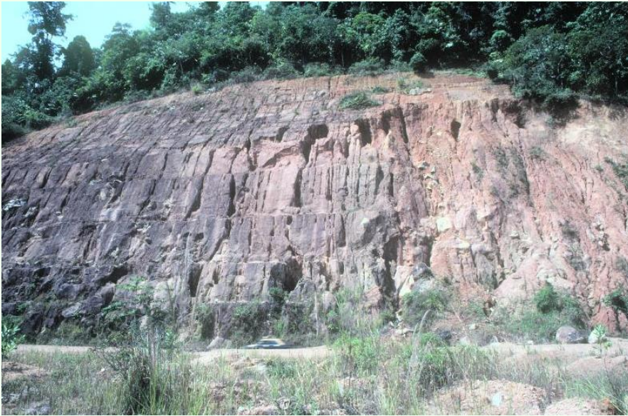
KL – Karak highway – erosion or slip?
