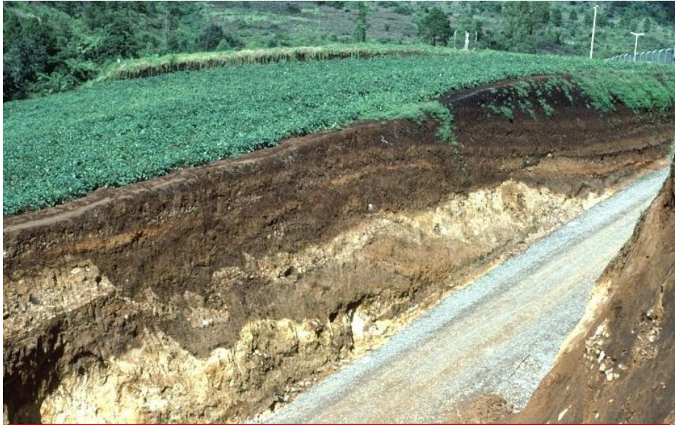
Darajat Geothermal Project slip on access road to base camp – soil conditions
